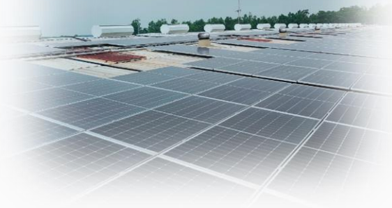
Roof-top solar at our Conductor plant in Orissa
