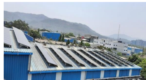
Solar Panels on White Oil Plant @ Rabale (Navi Mumbai)
