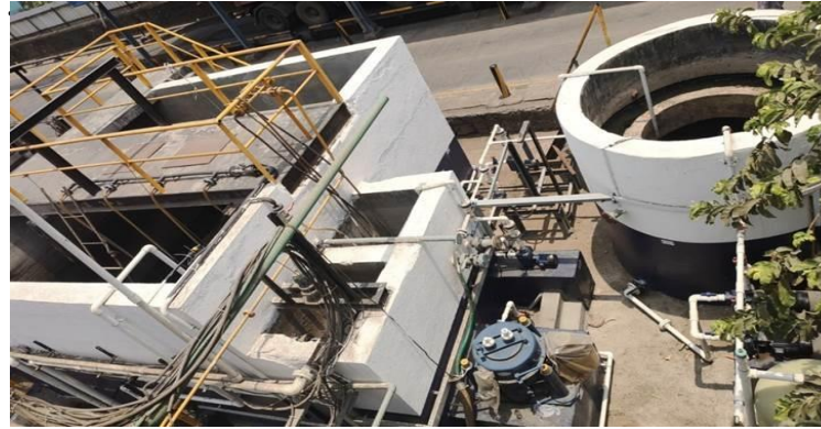
ETP plant at Rabale, Navi Mumbai
