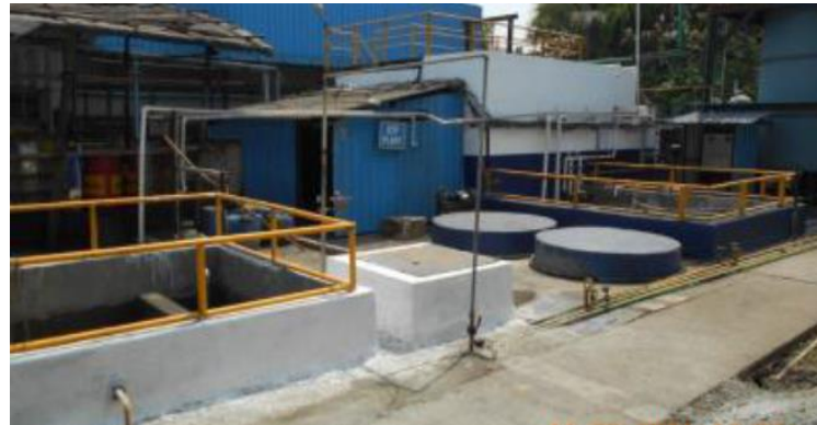
ETP plant at Rabale, Navi Mumbai
