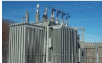
Transformer & Sp Oil
