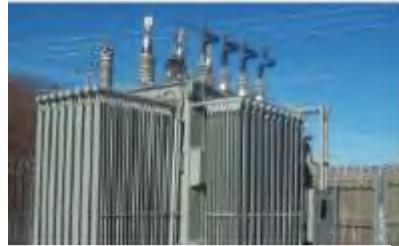
Transformer & Sp Oil
