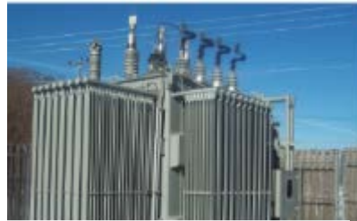
Transformer & Sp Oil
