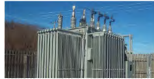
Transformer & Sp Oil
